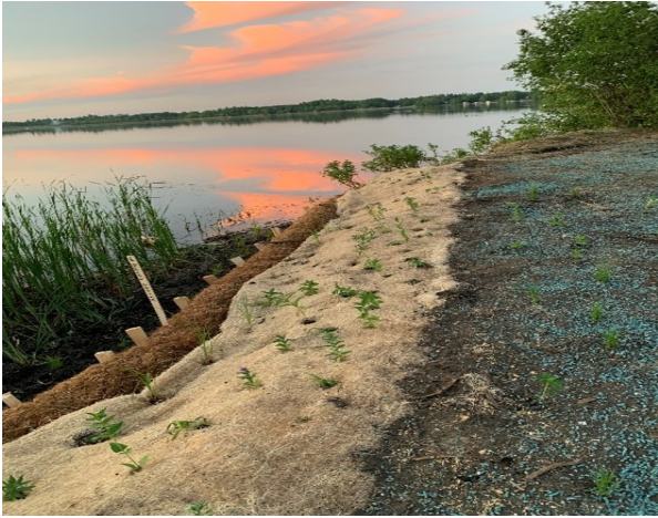
This is a shoreline stabilization project that was implemented in May of 2021.
